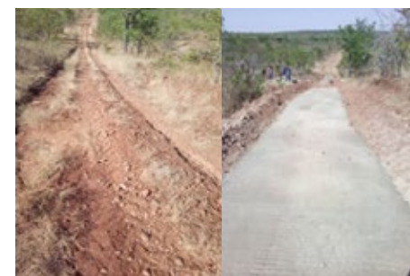
Before (left) and after (right) construction of the concrete hill ramp to Mvuvwe Picket
