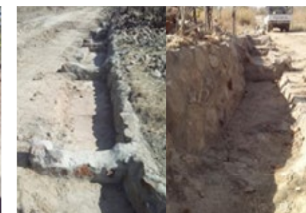
Check dams restrict and slow the flow of water run-off and erosion
