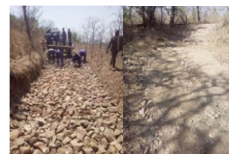
Before (left) and after (right) construction of the concrete hill ramp to Mvuvwe Picket
